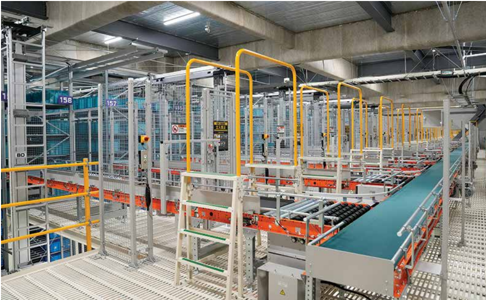
SB Logistics installed the conveyor and sortation system on a mezzanine level.
